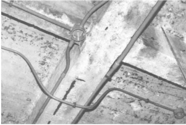
Figure 18-24 An installation with several bends in nonmetallic conduit. (Courtesy of Carlon Electrical Sciences, Inc.)
